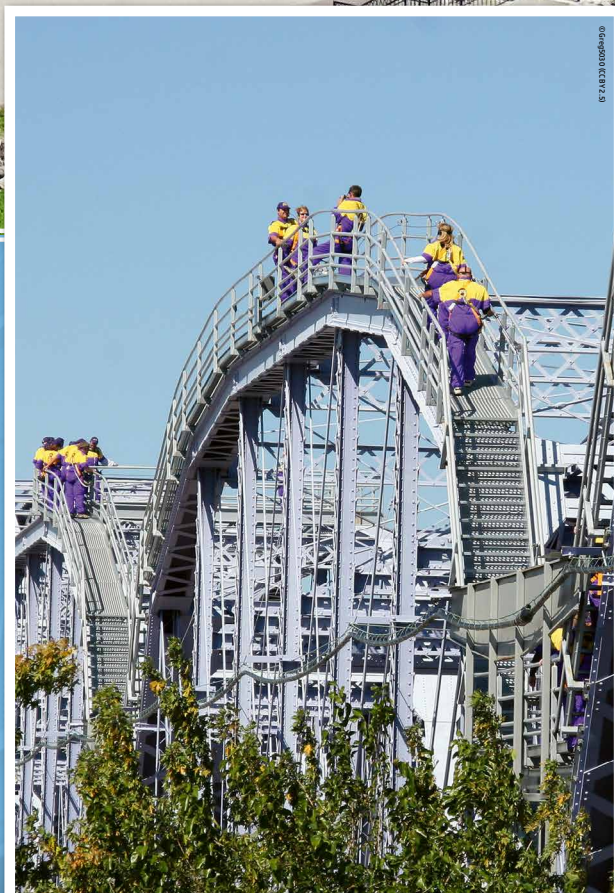
Maintenance walkway attached to bridge with Lindapter girder clamps
